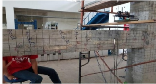
Fig. 6. Crack Pattern of STR-2
